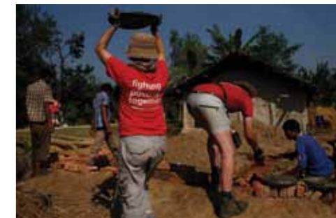
ActionAid volunteer Kezzie Zukas carries a tray of 'masala' (hand-mixed cement) as John Varian helps a local man lay bricks in Belarpur.
