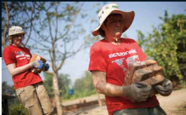
Volunteers Marjolein Atling (left) and Sue Pengilley carry bricks during ActionAid's First Hand Experience to construct 23 homes for the Kamaiya people in Belarpur village, Kailali, Nepal.
