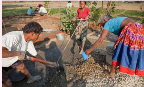
Shiva Tharu (left) works with his wife, Palti (centre), and his mother, Labhutti Tharu to make cement to build their new home.
