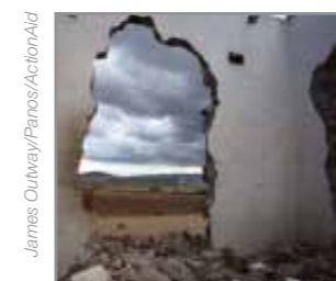
A demolished house near Ga-Puka.
